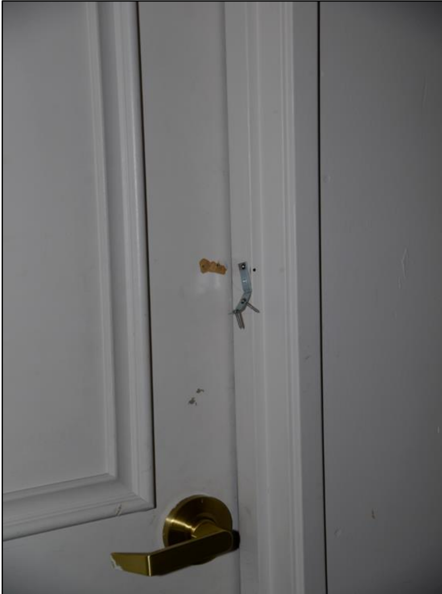
(Door leading to the stairwell secured by "L" bracket)
