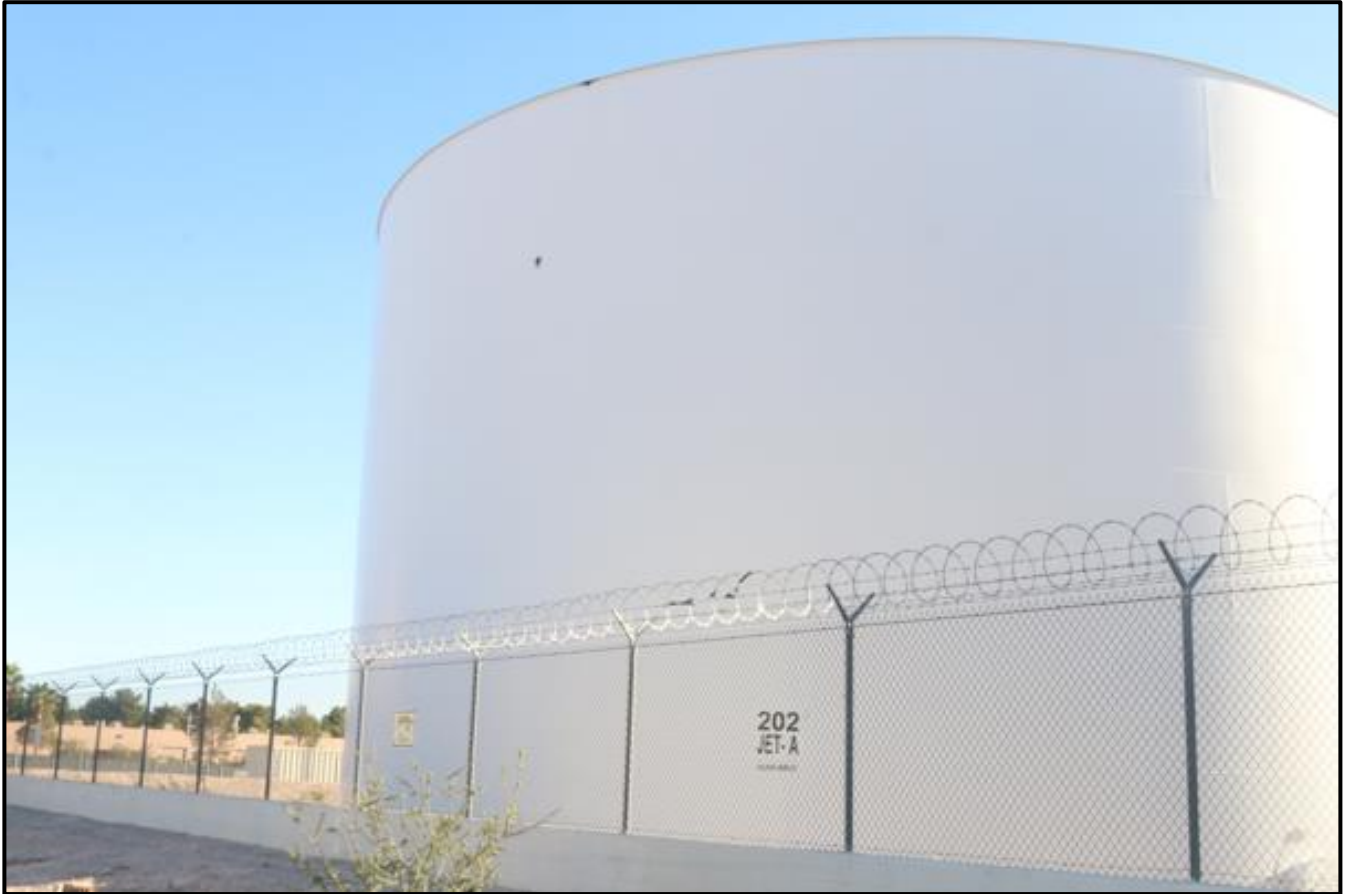
(McCarran International Airport fuel tank with bullet strikes)
